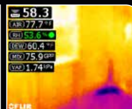
Corner moisture: Iron
