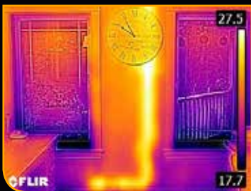
Pipe in wall Thermal Image with MSX
